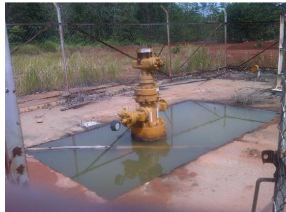
Figure 1 Well M-03 Condition
