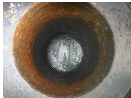
Figure 3 Stuck disk of the problematic lower master valve
