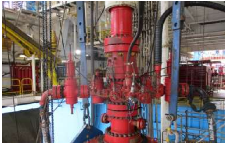
Figure 1: RCD Installed on BOP
