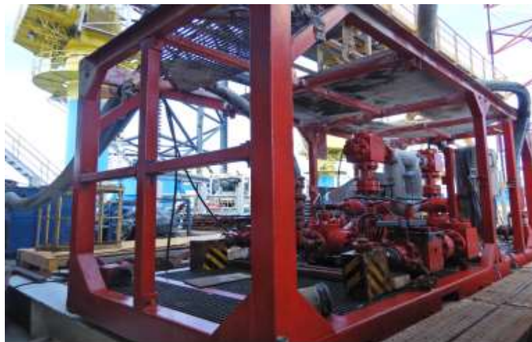
Figure 2: MPD Automatic Choke Manifold
