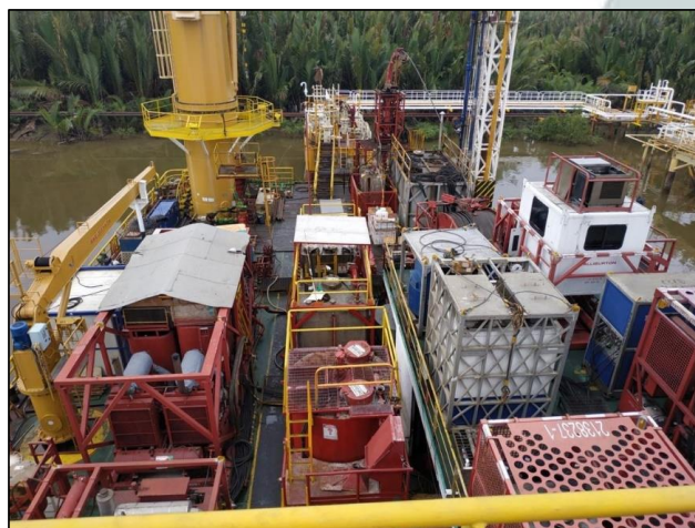
Figure 12. SCON activity on Well Intervention Barges
